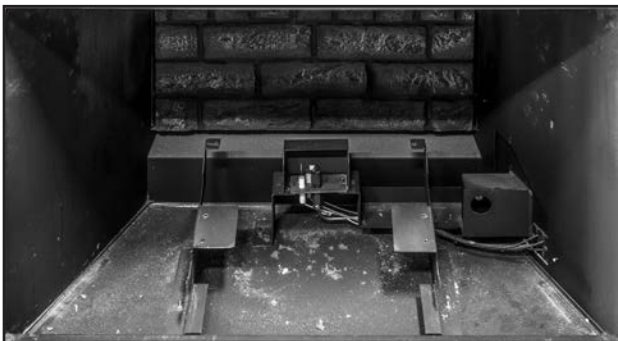
Figure 42: Lift the burner off the mounts and pull it out of the inlet box. The unscrew the panel brackets (T20's) from each side of the baffle to remove the left and right side liners.
